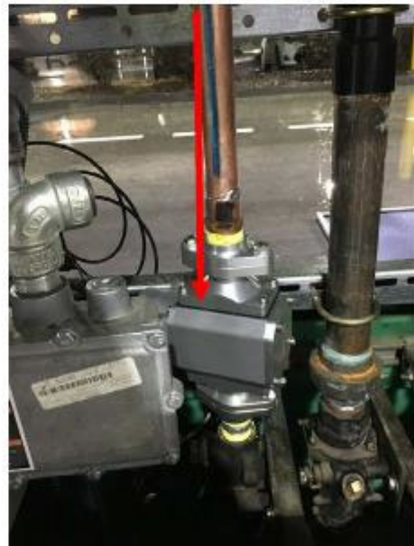
Figure 9: Install new Veeder-Root Balance Flow Meter.
