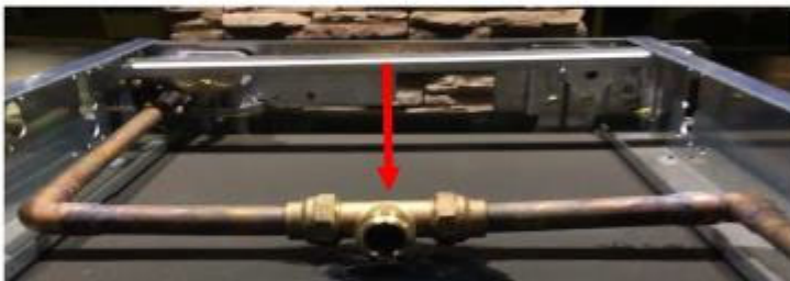
Figure 5: Fitting at top of existing Vapor Recovery Manifold in the Dispenser.
