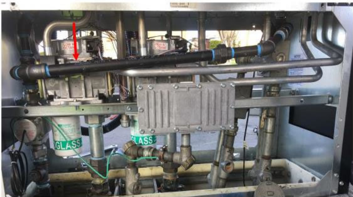
Figure 12: Galvanized Piping Configuration
