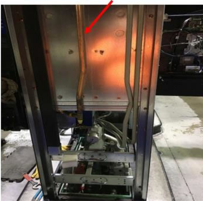
Figure 3: Existing Vacuum Assist copper Vapor Piping:
