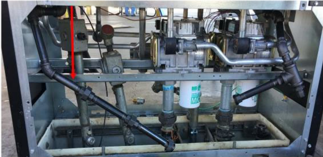
Figure 11: Galvanized Piping Configuration
