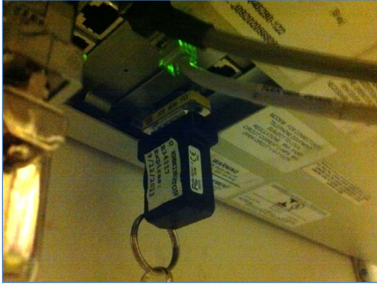
Figure 4: Maintenance Tracker Key Plugged Into TLS Console
