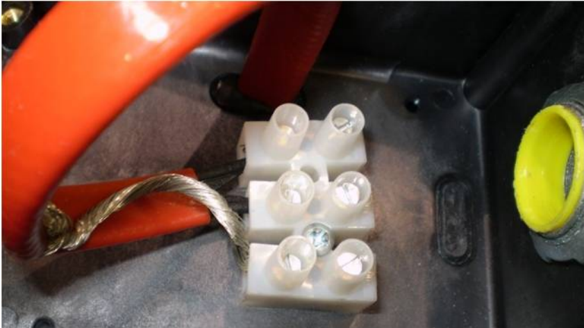
Figure 37: Termination block inside the electrical junction box
