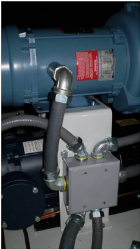
Figure 23: Blower electrical connection conduit
