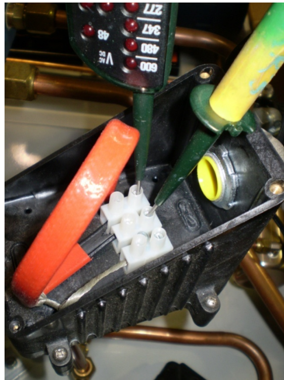
Figure 16: Heat Trace Circuit Test
