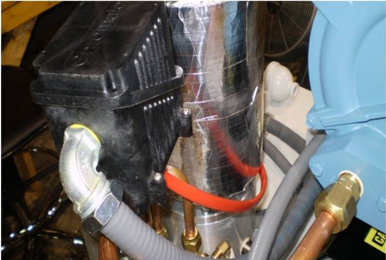
Figure 48: Installed electrical junction box with electrical connections
