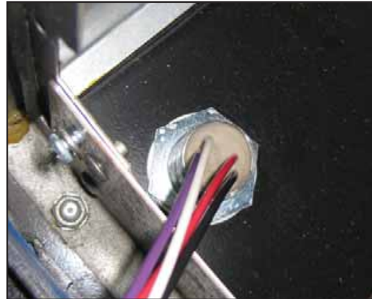
Figure 4: Potted Nipple Installed
