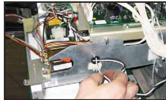
Figure 9: Power Harness Wiring
