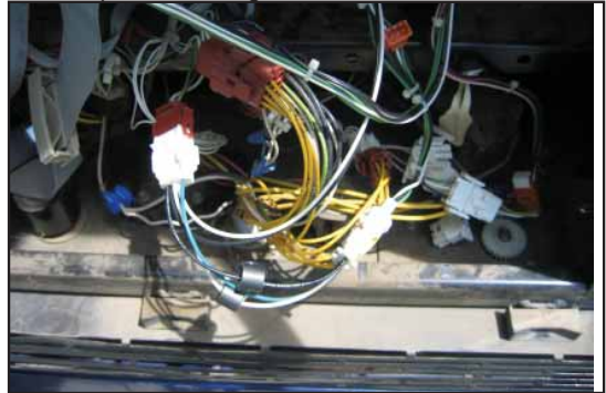
Figure 4: Power Distribution Wires
