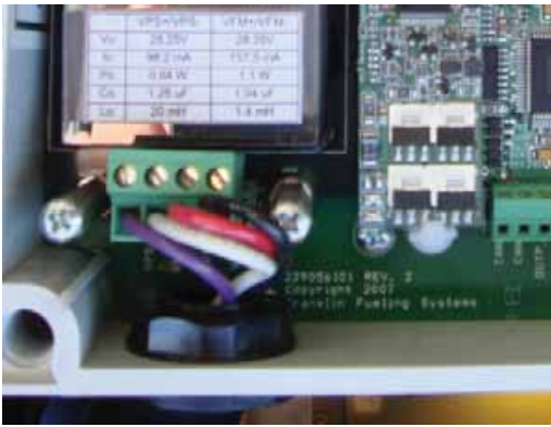
Figure 15: Wires Connected to DTU
