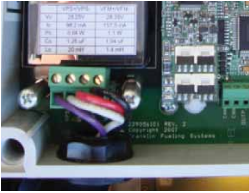
Figure 16: Wires Connected to DTU
