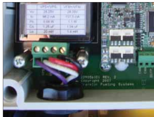
Figure 13: Wires attached to DTU
