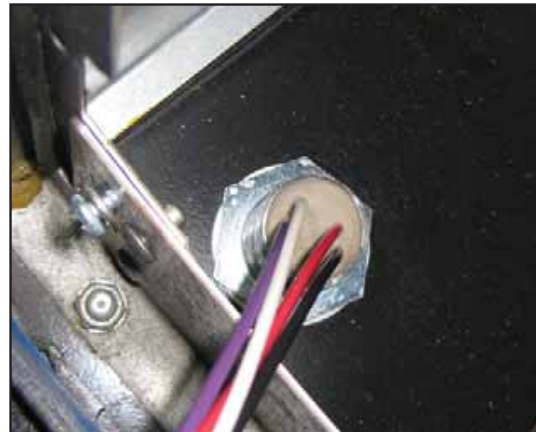
Figure 5: Potted Nipple Installed
