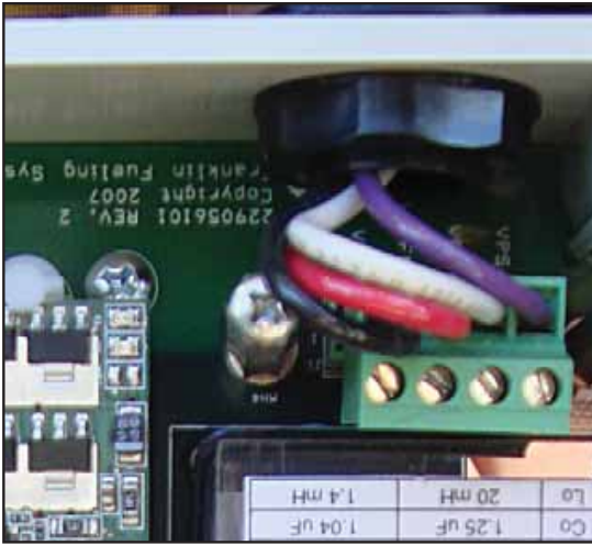
Figure 14: Wiring Connection to DTU
