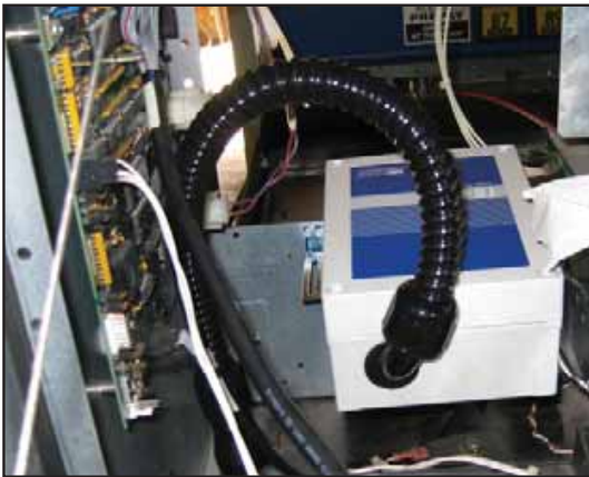
Figure 17: DTU Installed with Cover On
