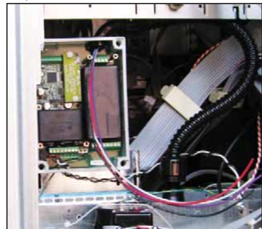
Figure 13: Wires in Flexible Conduit
