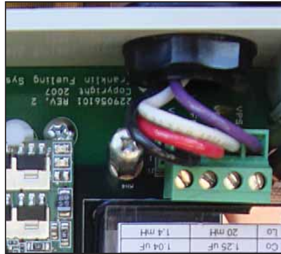
Figure 12: Wiring Connection to DTU
