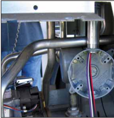
Figure 8: Junction Box Connected to Potted Nipple
