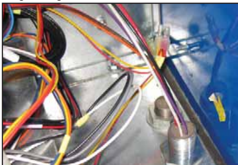
Figure 8: Potted Nipple Installed
