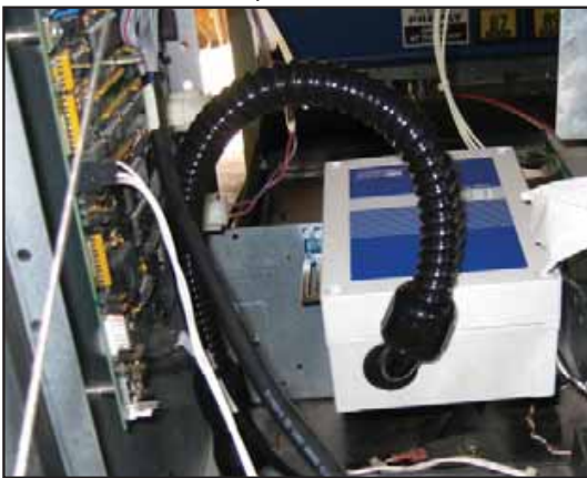
Figure 16: DTU Installed with Cover On
