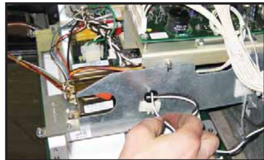
Figure 10: Power Harness Wiring
