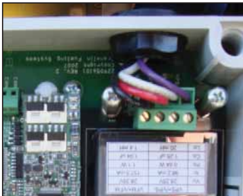
Figure 16: Terminal Block Wiring
