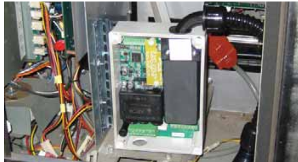
Figure 13: Reinstall Barrier Cover
