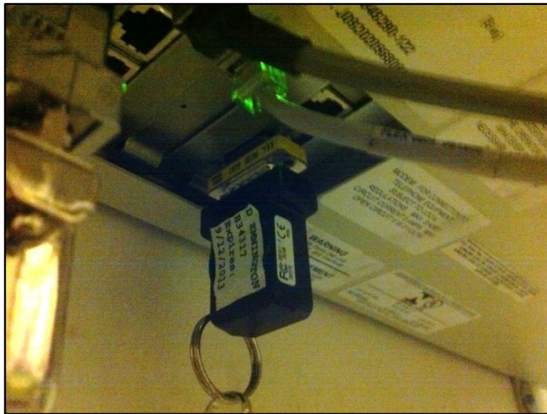
FIGURE 4 Maintenance Tracker Key Plugged Into TLS Console
